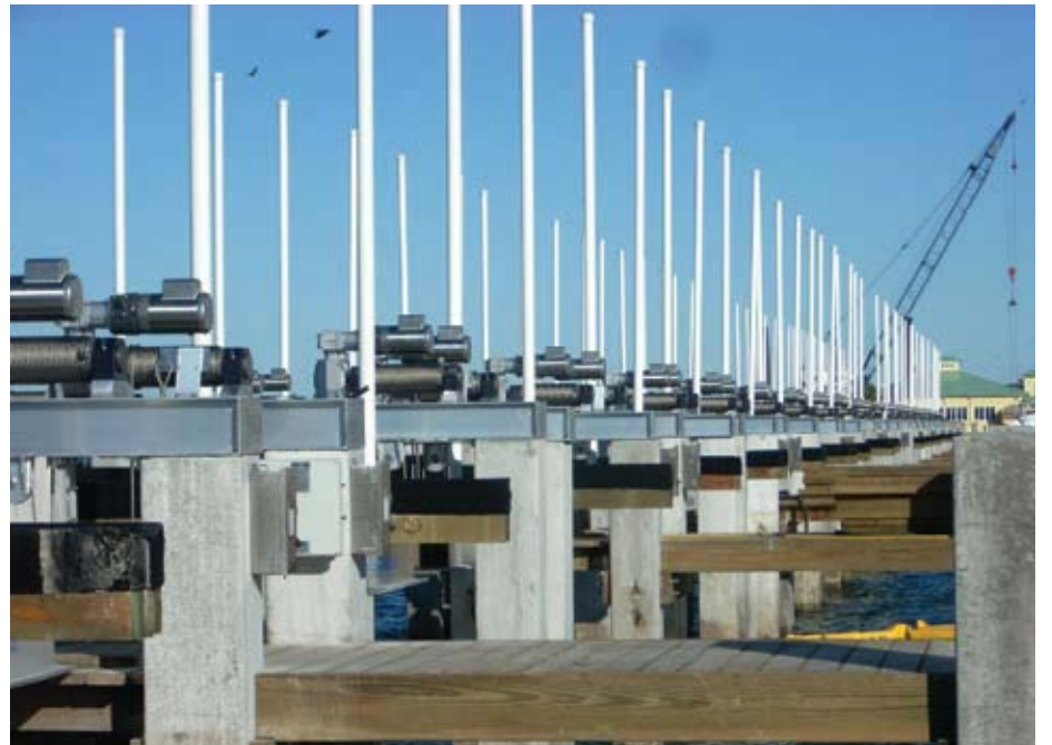
The Baldor District Office in Tampa supplied 105 Baldor-Reliance 2 HP Paint-Free motors for the installation at the new Bluepoints Marina in Port Canaveral, Florida.
